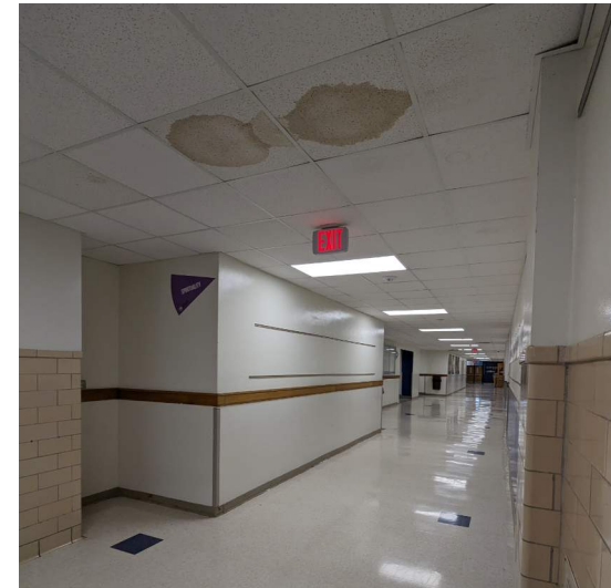
AREAS OF STAINED TILES
