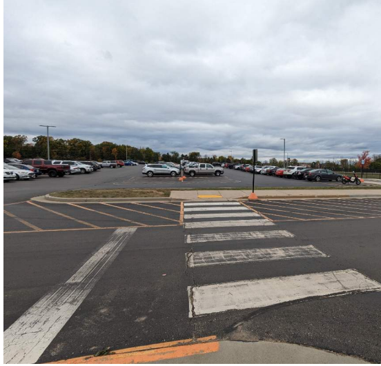
AREAS OF CRACKING ASPHALT
