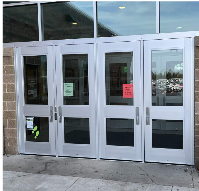
EXTERIOR DOORS LACK MONITORING
